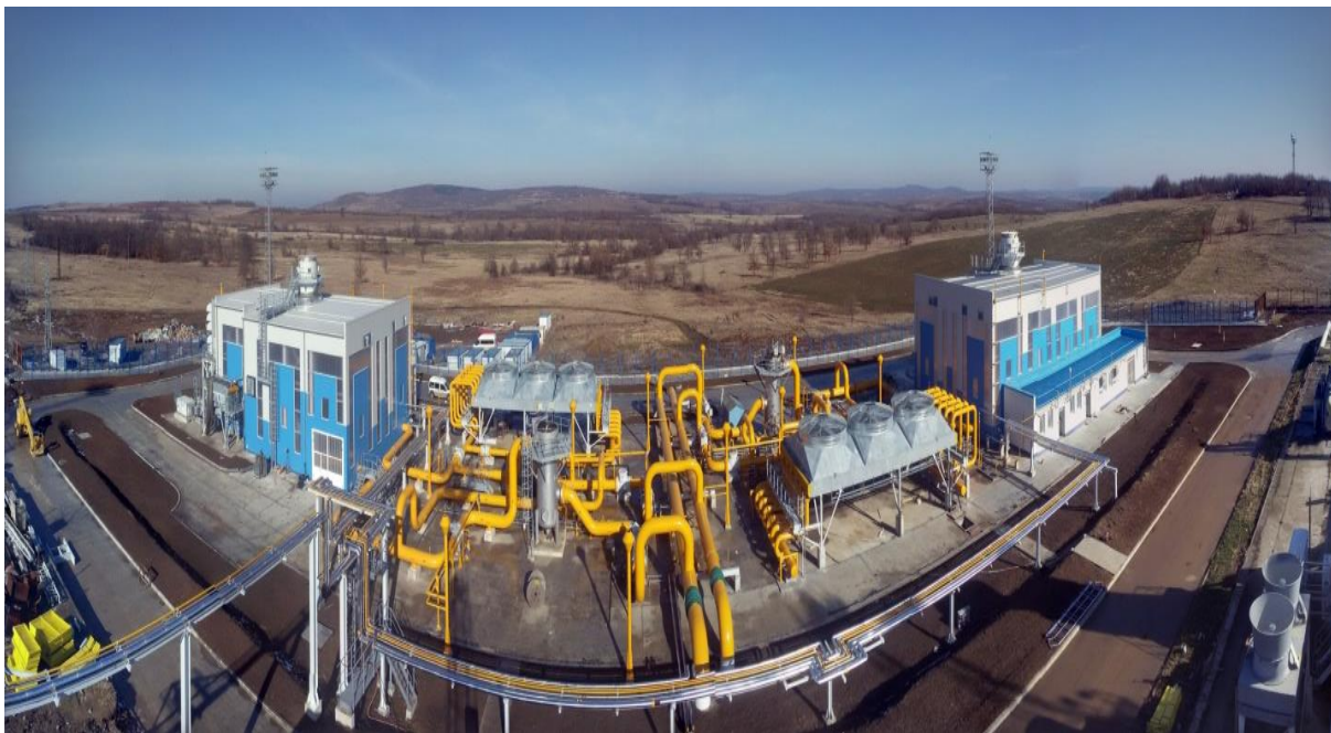
Compressor station Strandja
