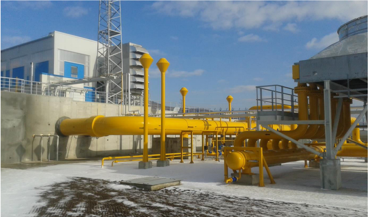
Compressor Station Lozenets
