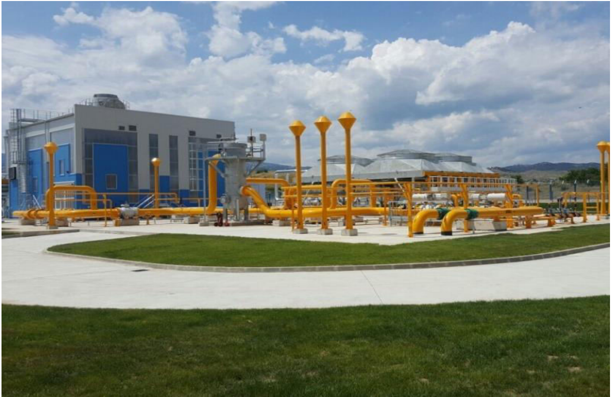
Compressor Station Ihtiman
