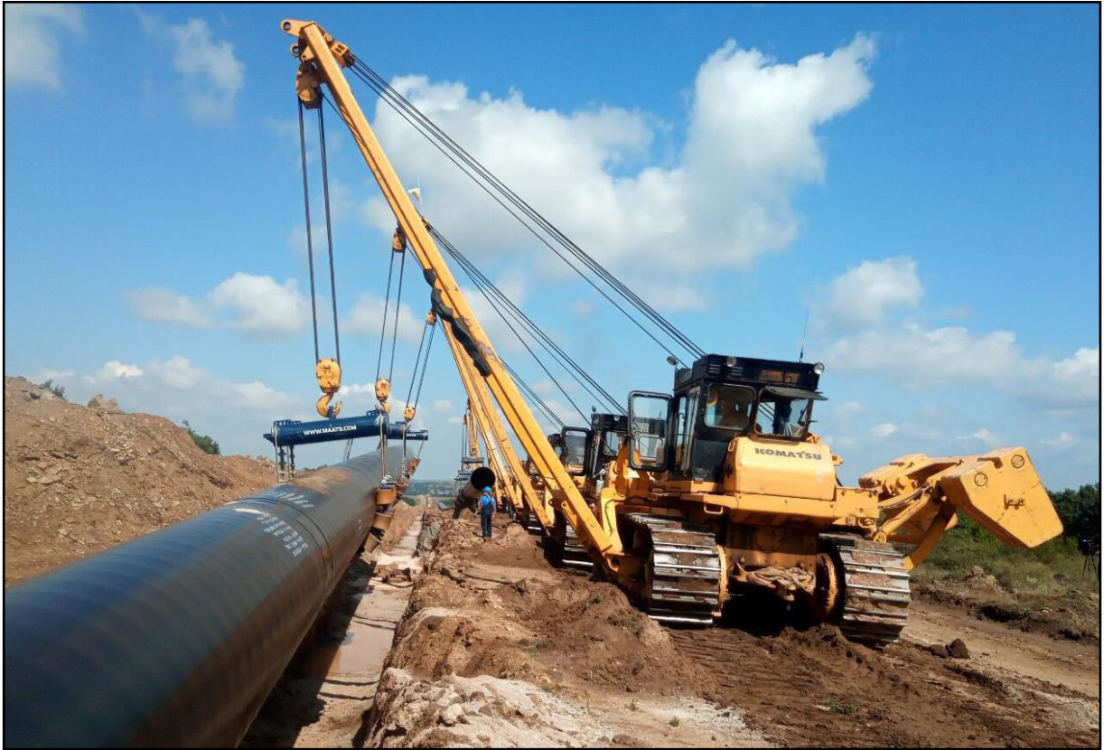
Construction of a pipeline network part of a high pressure gas pipeline
