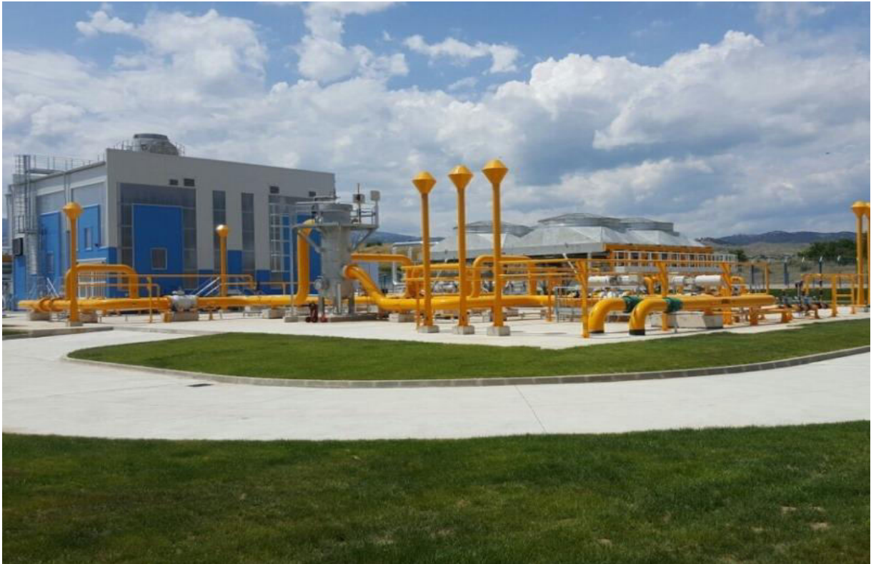
Compressor Station Ihtiman
