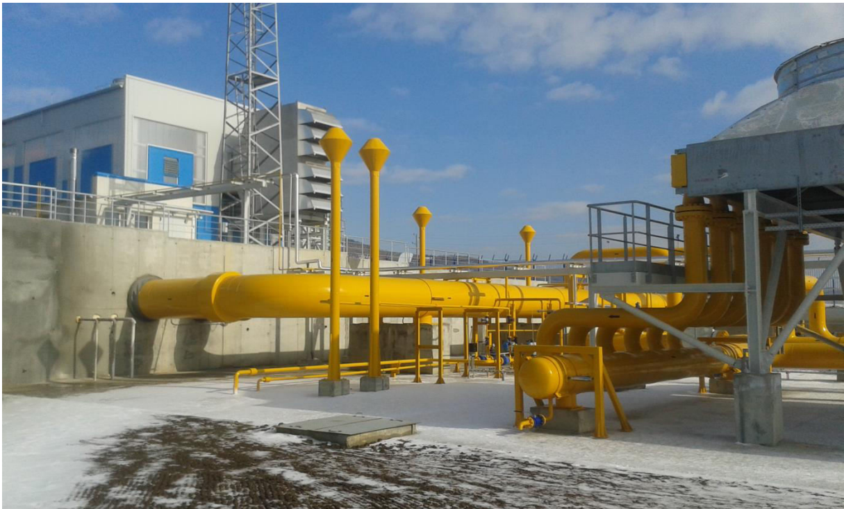
Compressor Station Lozenets
