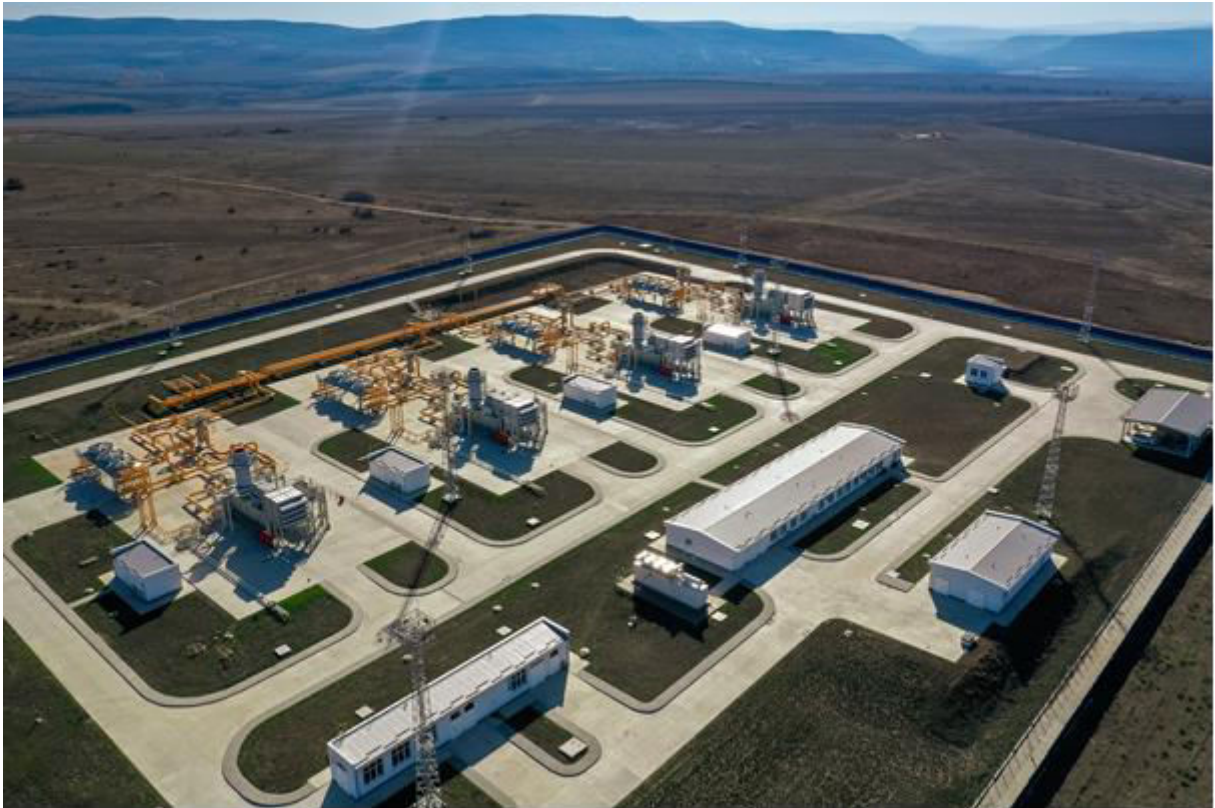
Compressor Station Nova Provadia
