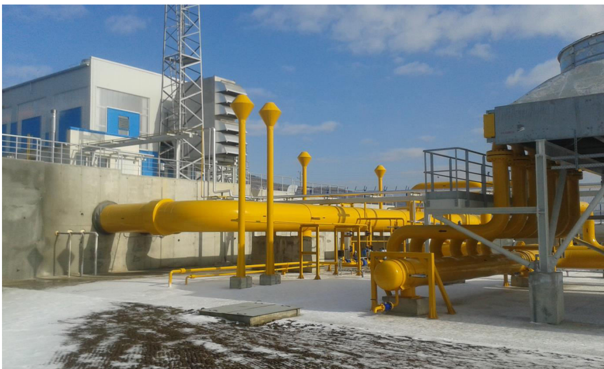
Compressor Station Lozenets
