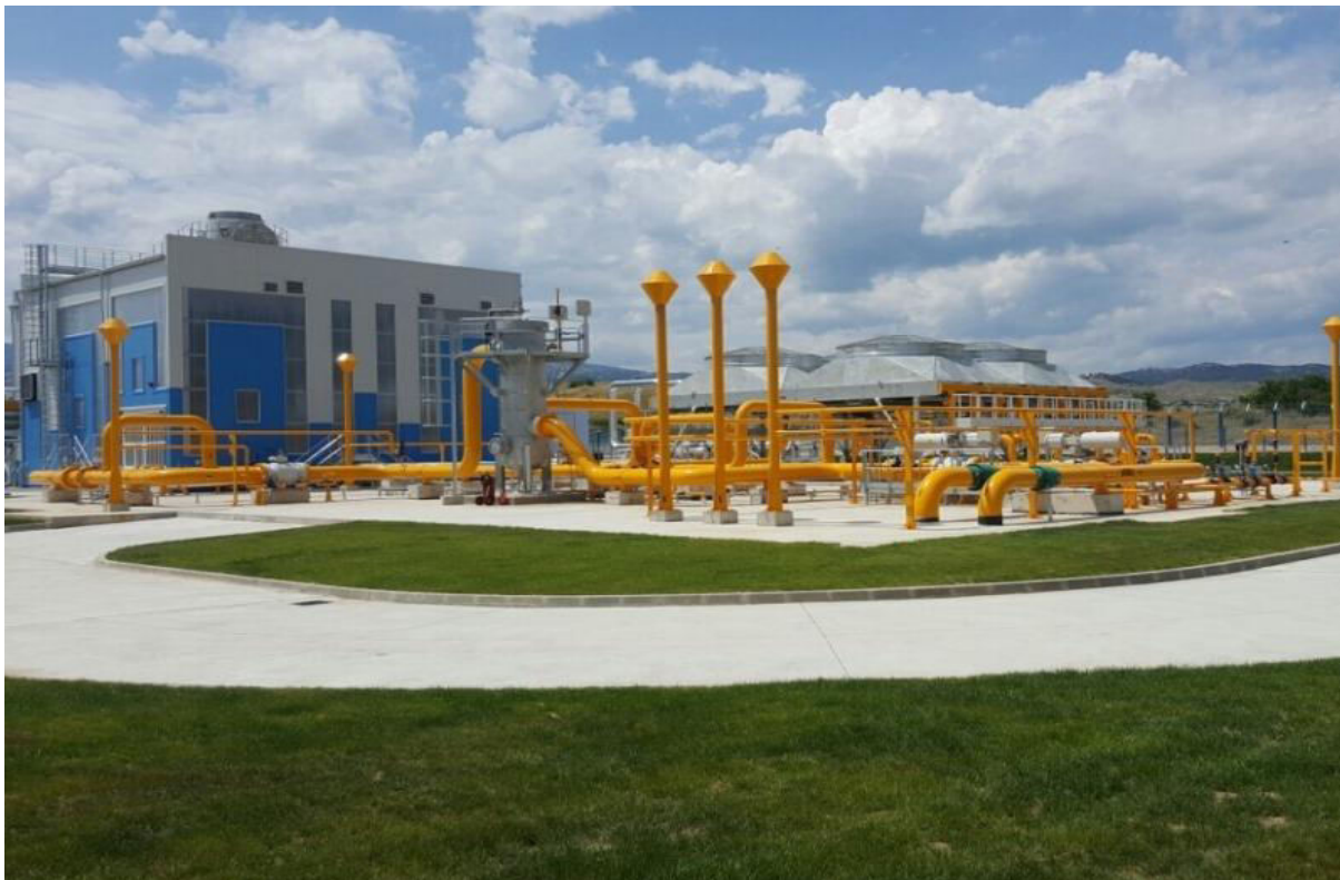
Compressor Station Ihtiman
